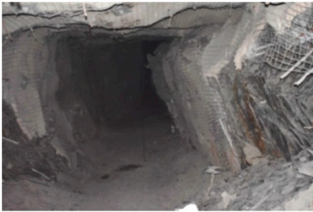
Fig. 27. Buckling and tensile fractures in tunnel sidewalls due to anisotropic rock mass aligned with foliation, driven by stress concentration, rotation, and poor rock quality in shear zones in CSA Mine in Australia [291].
