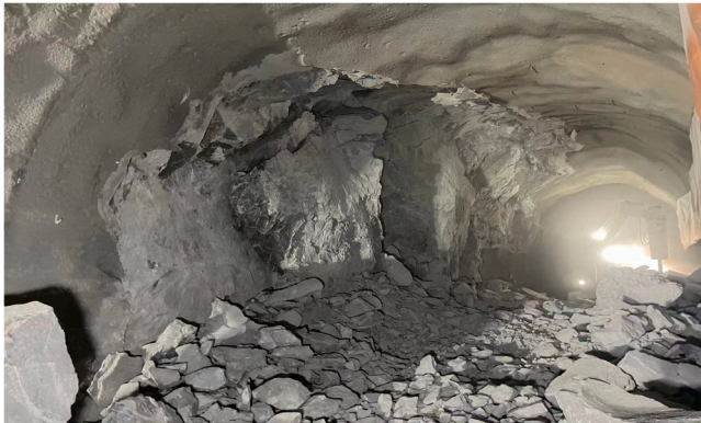
Fig. 9. Structural planes in the extremely intensive time-delayed rockburst.
