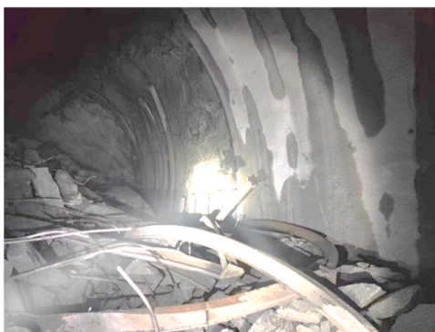
Fig. 1. Intensive spatial-temporal delayed rockburst in a tunnel in south-west China.
