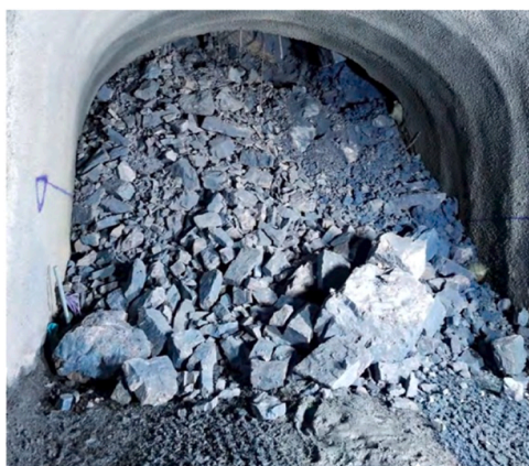
Fig. 15. Collapse failure in the underground caverns [22].
