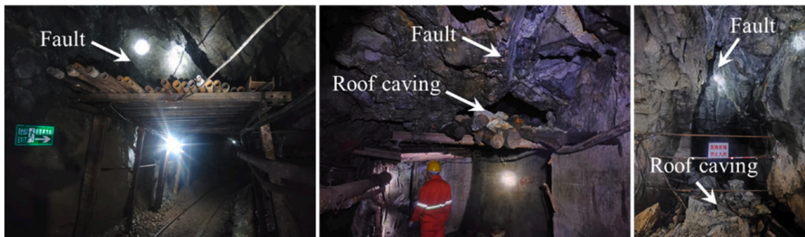
Fig. 9. Rock mass fracture and caving in fault zone.
