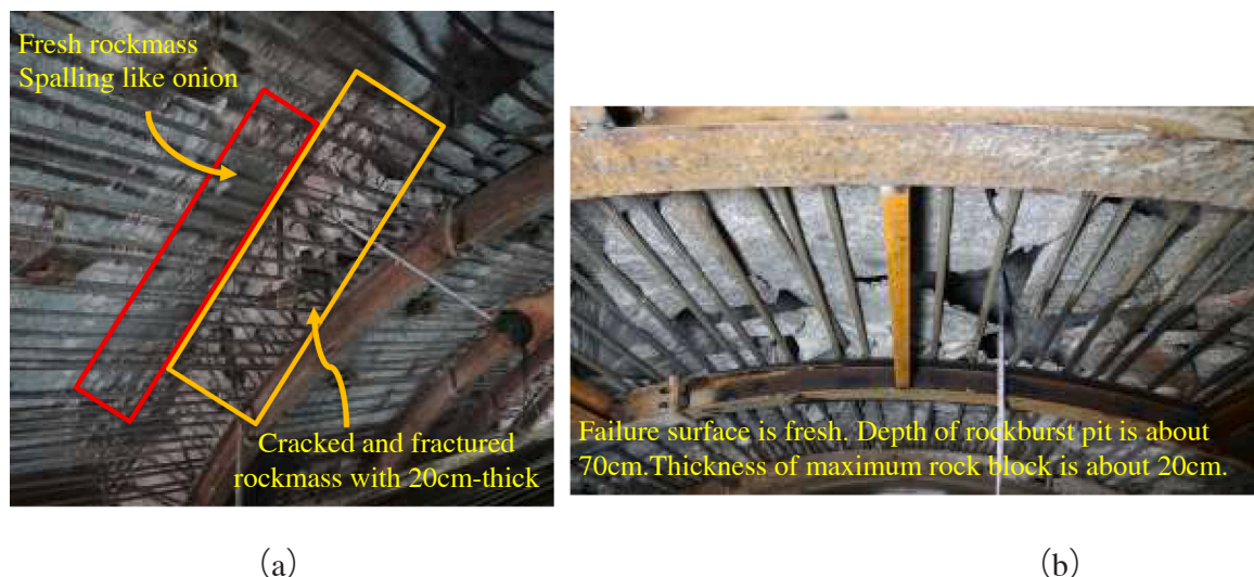
Fig. 17. Slabbing and slight rockburst in the tunnel in Xinjiang Province under high stress. (a) Slabbing in the left vault, (b) Slight rockburst in the upper vault.
