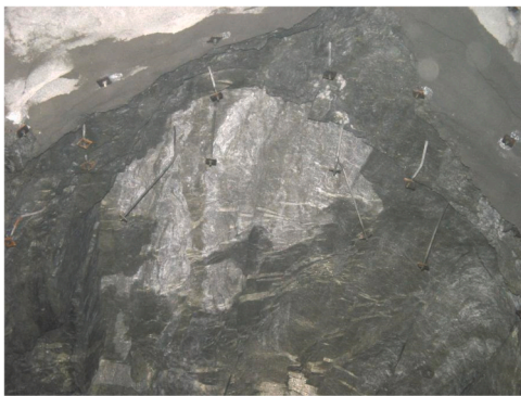
Fig. 4. Spalling on the roof of Slice 1 in SL1.
